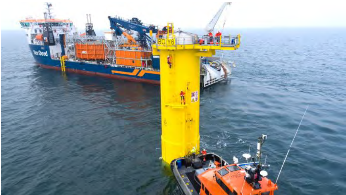
Figure 30: Van Oord's Nexus Cables ship installing cable at a wind turbine monopile
